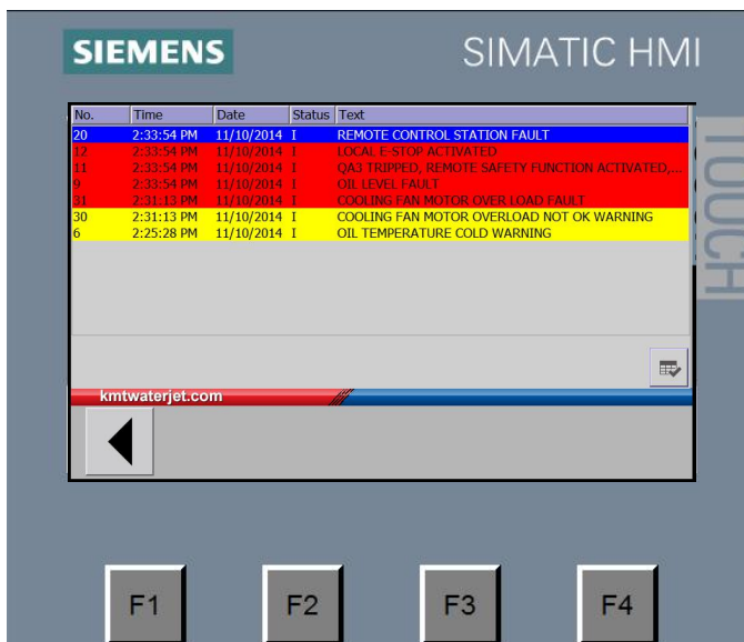
Figure 4-8: Alarm History Screen
